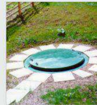
Sewage Treatment Plant
